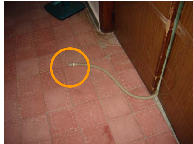
Used anaesthetic gases pumped into main theatre corridor
